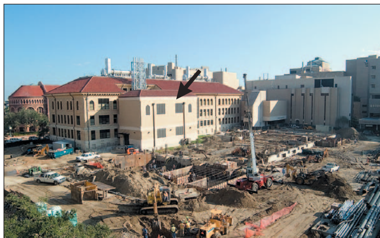
The Galveston National Laboratory under Construction on the Campus of the University of Texas Medical Branch, October 2005.
